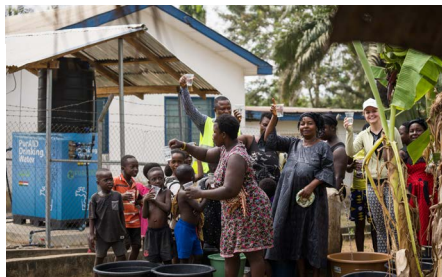
Modular, mobile, pallet-based water purification equipment installed in Akim Wenchi settlement, Ghana Disease causing bacteria, iron and manganese impurities removed from the water
