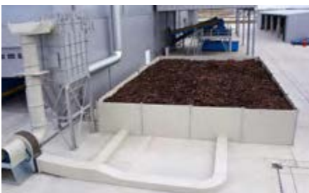
Air treatment project at a waste management centre, Subotica, Serbia Capacity: 20,000 m 3 /h
