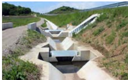
Stormwater treatment at the Lugoj-Deva highway, Romania ENVIA TRP oilseparators were installed
